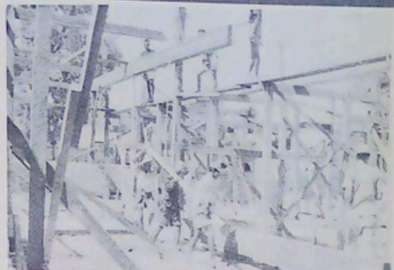
Raising the timbers of the Revival Center. The language barrier and lack of building aids made it very difficult for Bro. Price and Bro. Hall to work with the natives.
